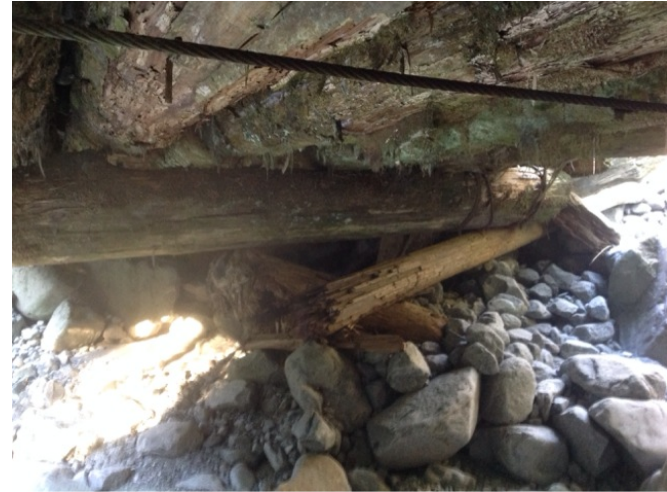
needle beam loose and material wedged under upstream
