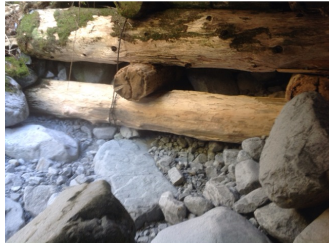
left abutment upstream scour
