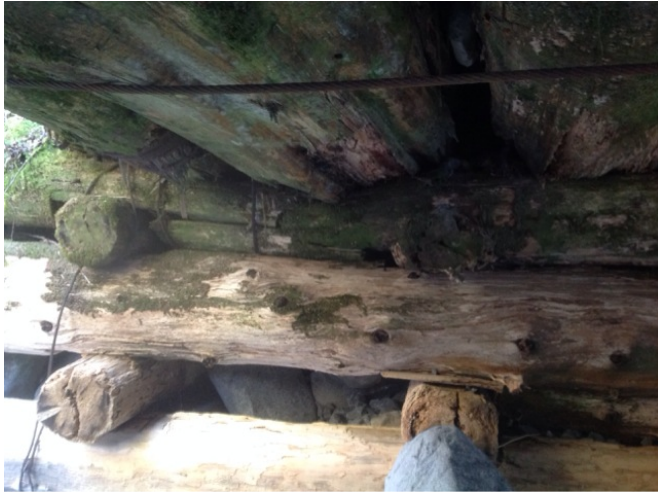
left abutment upstream top crib log crushing
